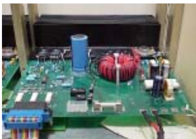
DUT Power Supply being assembled into the chamber. Opto isolation control section, DC-DC converter and linear output section are visible
